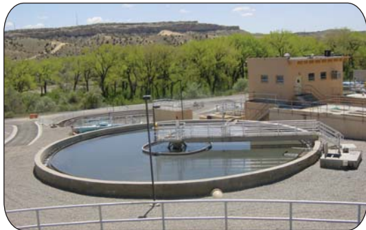
The City of Farmington Wastewater Treatment Plant
